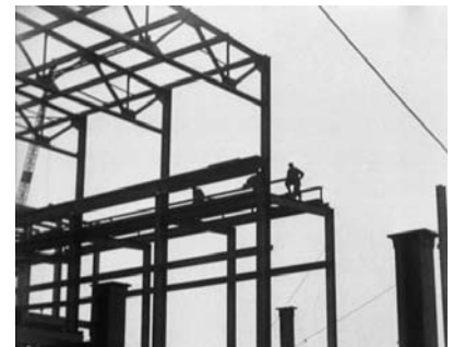
Construction of the Seaboard Paper Company Mill (1930), footage documenting the company's factory in Bucksport, Maine, preserved by Northeast Historic Film in 2015.
